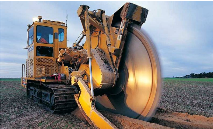
Leighton's Nextgen will roll-out 6,000ks of new fibre backhaul links, duplicating existing capacity.
